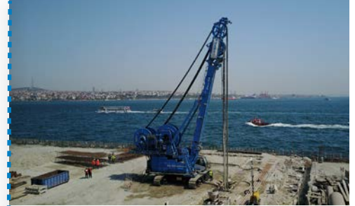
Diaphragm wall with HYDROMILL: 50,000 m 2 , 1200 mm thick panel to the maximum depth of 39 m.
