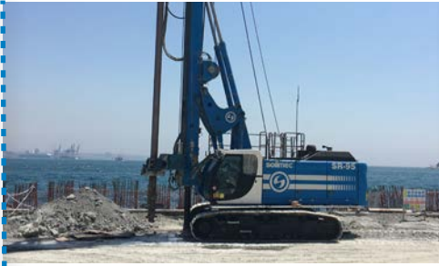
Deep Soil Mixing (by Turbojet®): 250,000 m 3 , Ø 1500 mm columns to the maximum depth of 28 m.
