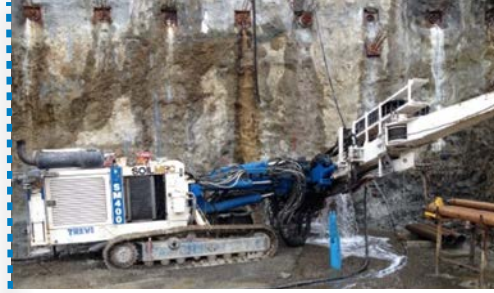
Temporary Ground Anchors: 30,000 m, Ø 165 mm anchors to the maximum depth of 30 m.
