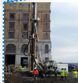
Jet Grouting bottom plug: 45,000 m 3 , Ø 2000 mm columns to the max depth of 29 m.
