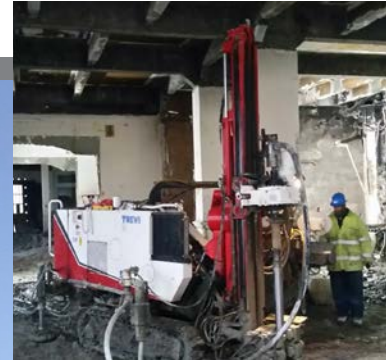
Jet Grouting (from inside): 40,000 m 3 , Ø 1500 mm columns to the maximum depth of 22 m.
