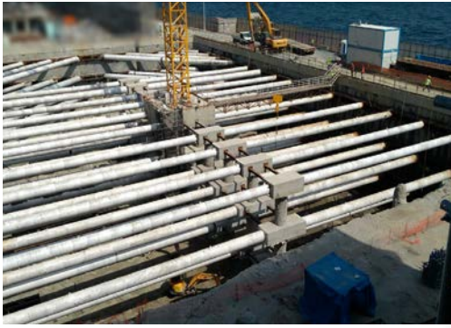
Mass excavation (100,000 m 3 ), Steel strutting (200 struts, 1500 t) and Dewatering by deep wells.
