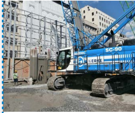
Diaphragm wall (Mechanical Grab): 18,000 m 2 , 1000 mm thick panels to the maximum depth of 35 m.
