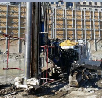
Micropiles (permanent): 10,000 m, ø 250 mm micropiles to the maximum depth of 26 m.
